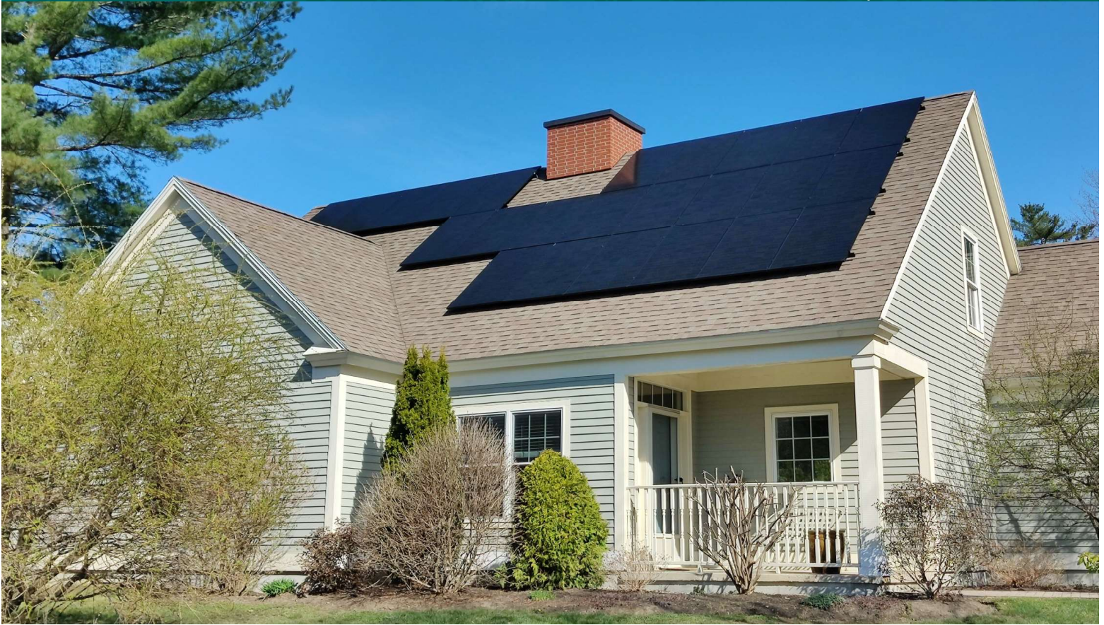
New solar panels top a Whipple Farm cottage at OceanView. (Photo taken April 2023)
