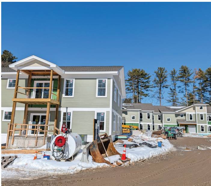
Evergreen Commons under construction; Building C is in the foreground, Building B in the background. (02/27/26)
